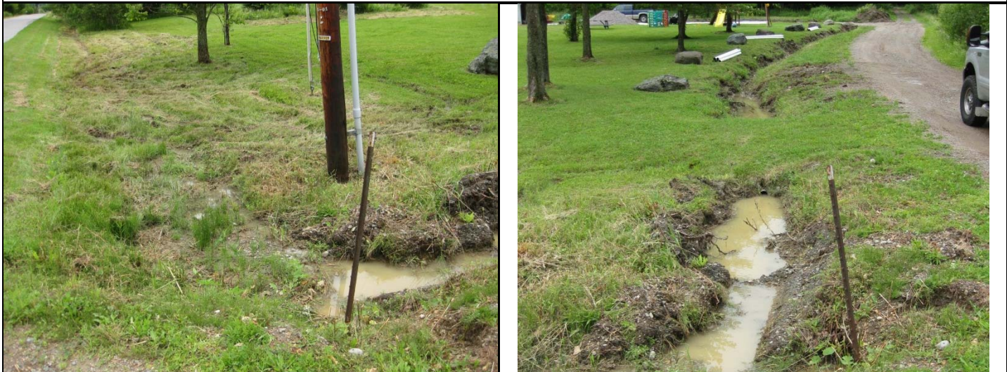
Photo 1. Water ponding along Old Stage Road at the intersection with Amber Lane Photo 2. Water ponding along Amber Lane
