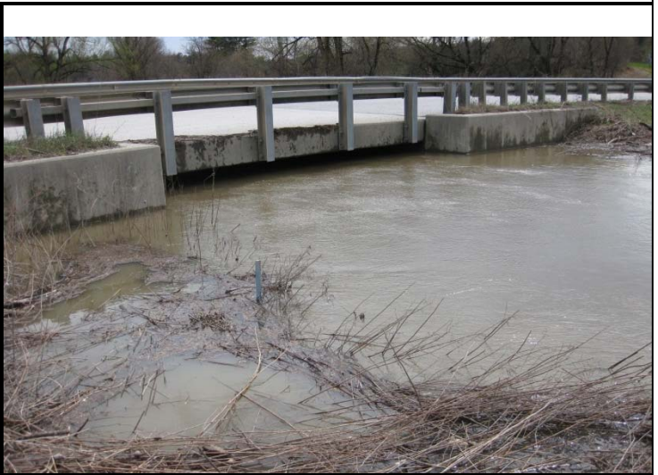
Photo 2. Downstream view of River Cove Road bridge during flood stage (4/28/2012)
