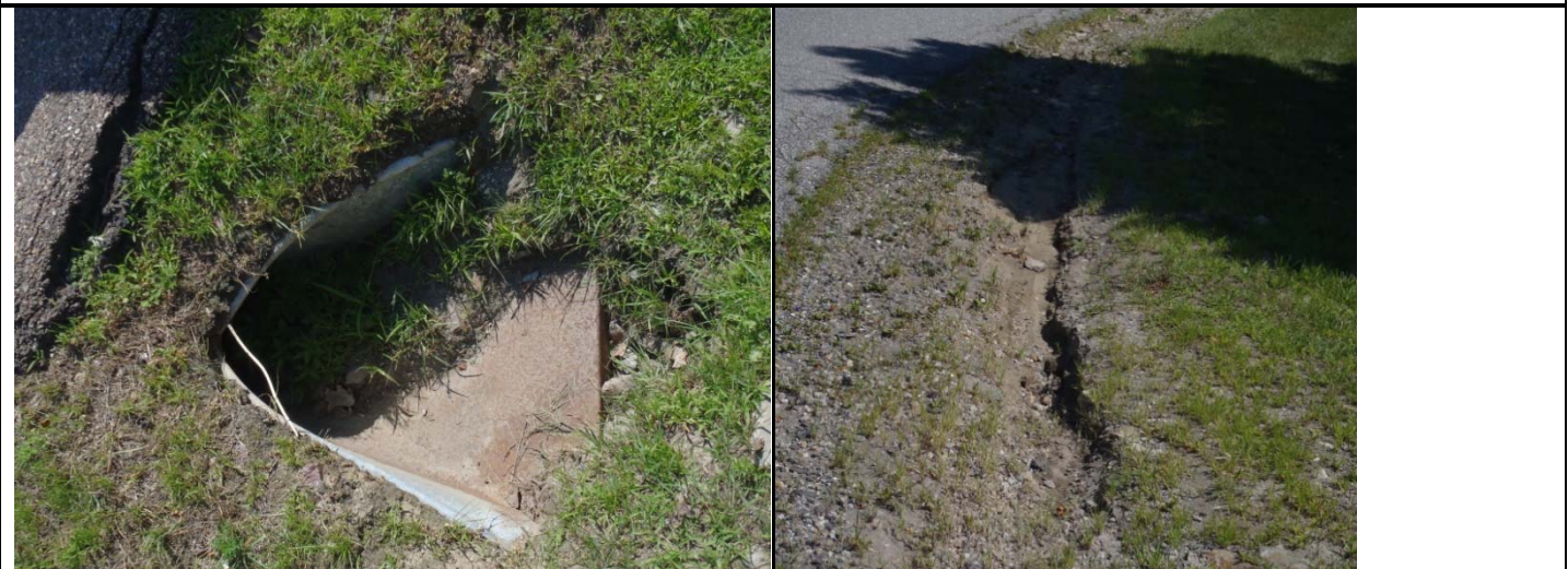
Photo 1. Culvert, beginning to be undermined
