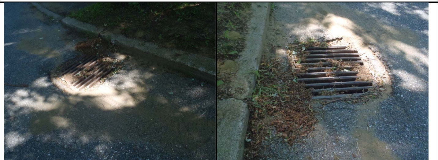
Photo 1. Clogged catch basin Photo 2. Debris accumulated at catch basin inlet
