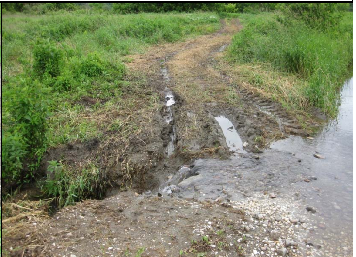
Photo 2. Erosion occurring at the discharge point.
