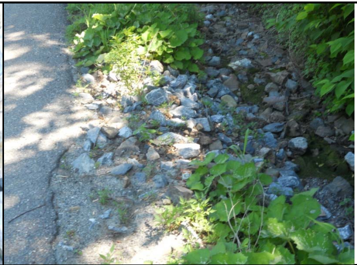
Photo 2. Road side erosion
