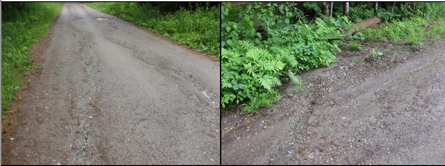
Photo 1. Erosion in the roadway. Photo 2. Sediment discharge along road shoulder.
