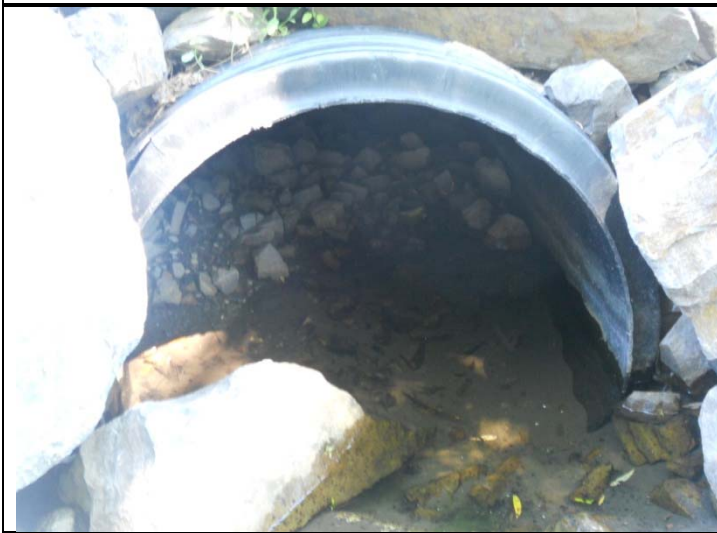
Photo 1. Aggradation in culvert.
