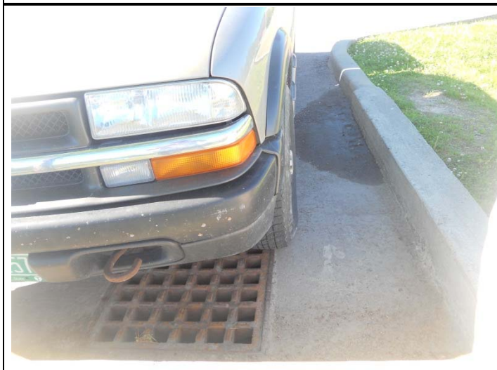
Photo 1. Water seeping from ground
