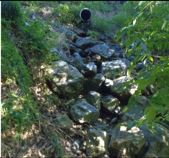
Photo 1. Erosion left of riprap
